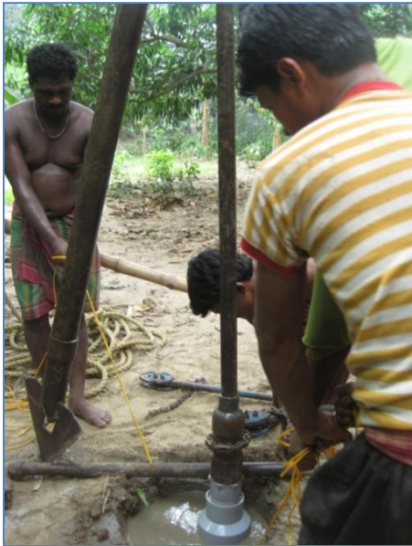
Figure 9: Lowering of the assembled 3m by 25cm PVC pipe into the 46cm by 9m hole
