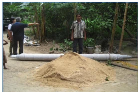
Figure 11: The 3m - pvc pipe with reducers at either end. The coarse sand in the foreground will be used to fill up the annular space around the pipe once the pipe is inserted
