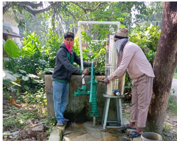
Figure 6: Maintenance of the filter at PW55
